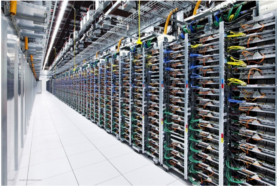
Google data center
